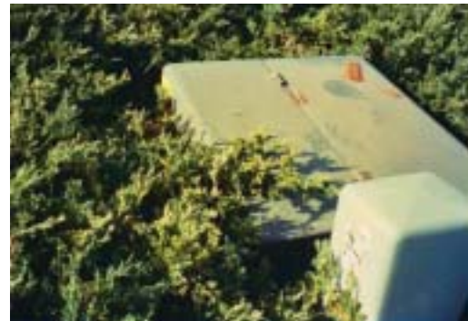
Top photo: Pad mount transformer hidden by landscape rocks and shrubs.
